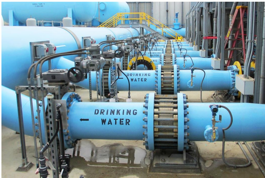
Around 500 AUMA actuators prove their worth in extreme environmental conditions at the Carlsbad Desalination Plant in California. Source: AUMA
