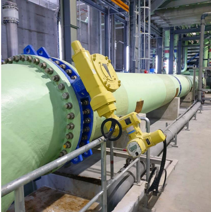
At the Keppel Marina East Desalination Plant in Singapore, 156 AUMA actuators are in operation across all treatment stages. Source: AUMA
